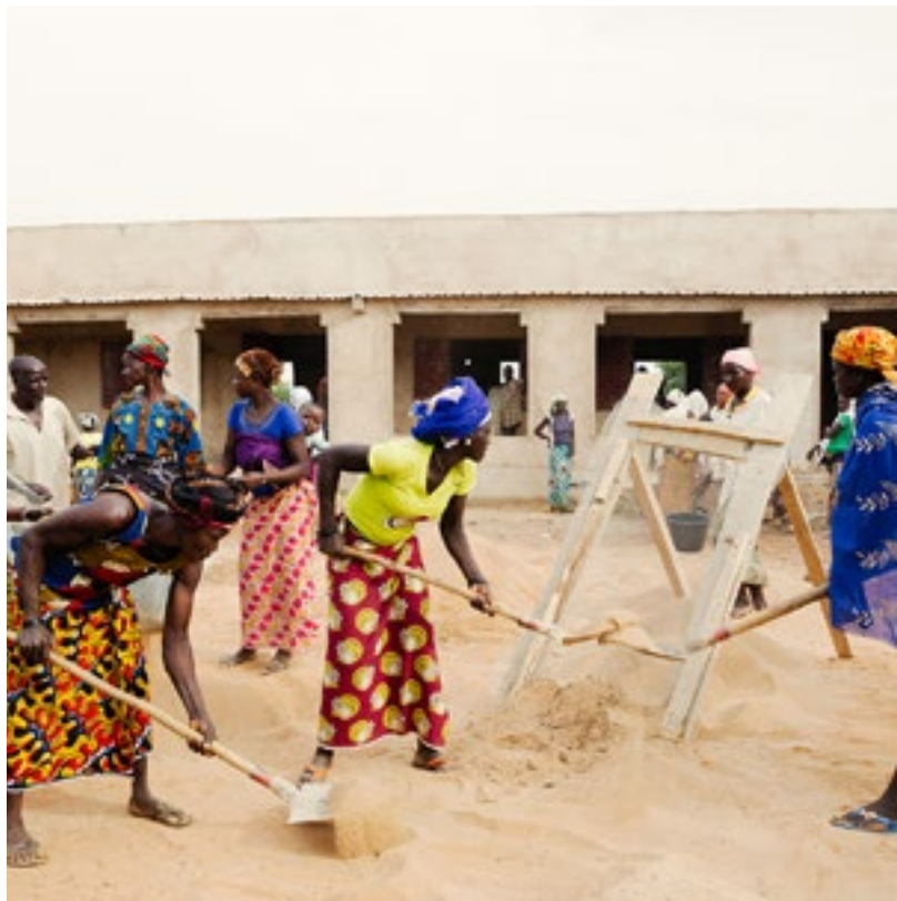
Women on the worksite building a new school in Burkina Faso. Photo: buildOn
